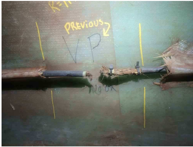
Figure 3-1 Turbine T01 (blade 107) 2020 LPS damage at 0.5 m distance from the root
